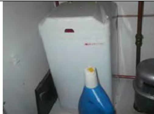
Modern non ACM water heater
