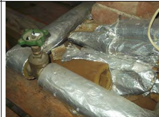
MMMF insulation to pipes with foil wrap. Non ACM
