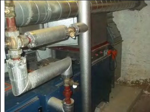
General view of Plant Room. Presumed asbestos gaskets, ropes and seals to plant Chrysotile
