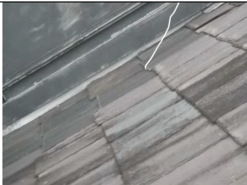
Strongly Presumed cement roof slates intermixed with natural slates
