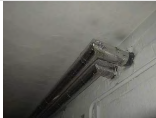
Plastered ceiling and foil wrapped MMMF non ACM lagging to pipes
