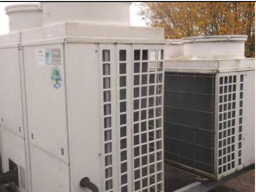
Presumed asbestos gaskets, ropes and seals to plant Chrysotile
