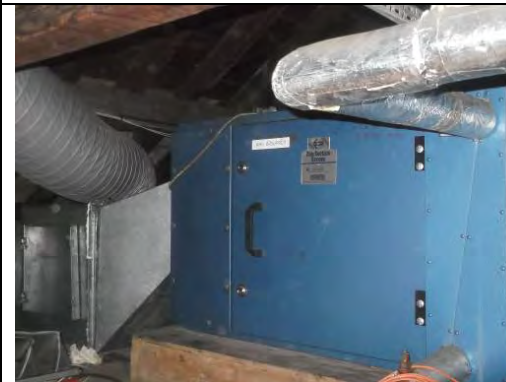
Presumed asbestos gasket, ropes and seals to plant
