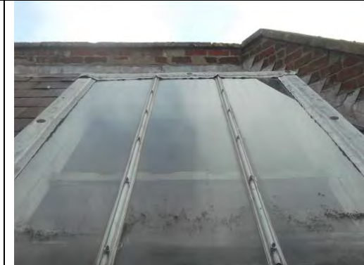
Presumed asbestos rope seals to roof lights Chrysotile
