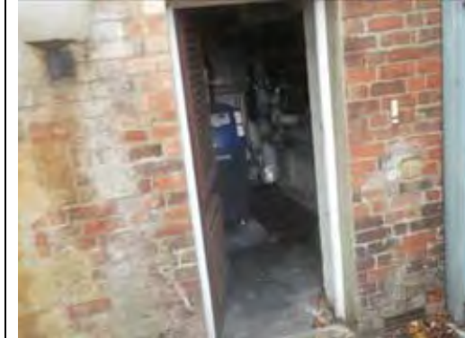
General view of Boiler Room
