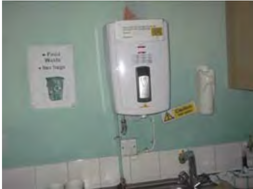
Modern non ACM water heater
