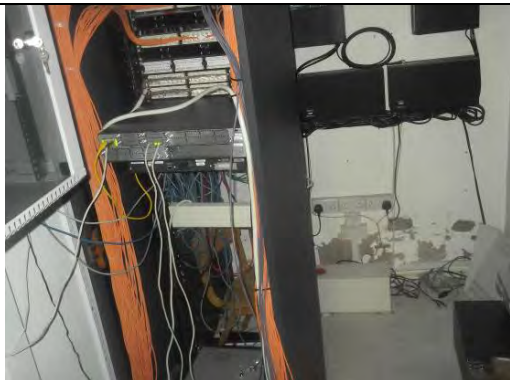
General view of 36. Comms Room
