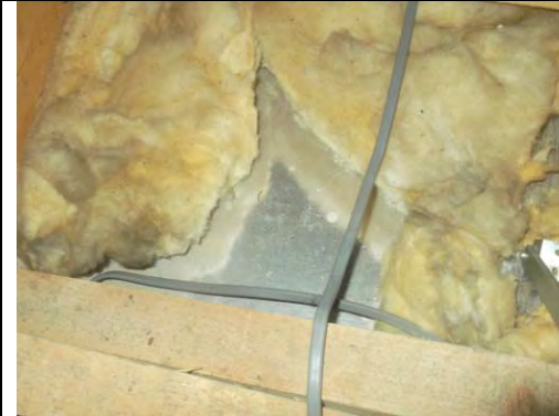
Modern non ACM MMMF insulation
