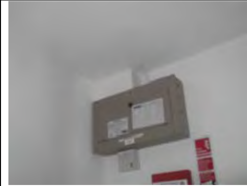
Modern non ACM electrics
