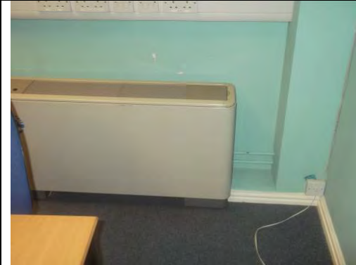
Modern non ACM air conditioning units/ heaters
