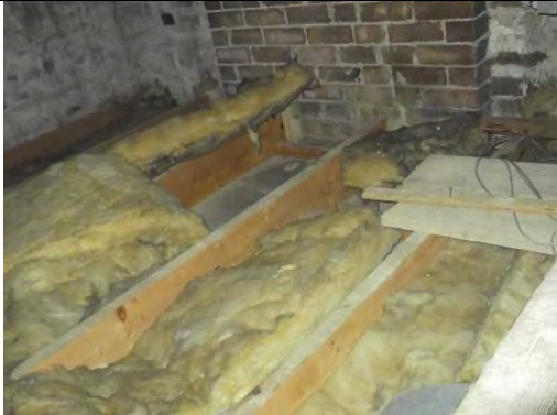
MMMF modern non ACM insulation
