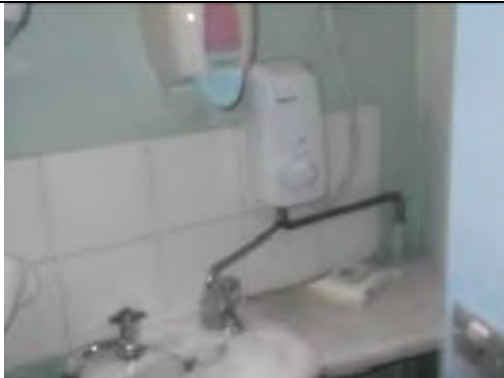
Modern non ACM water heater
