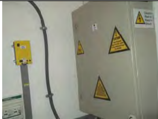
Modern non ACM electrics
