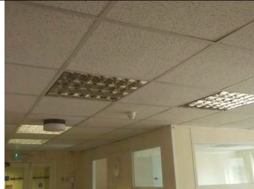
Modern non ACM suspended ceiling tiles and painted plasterboard walls and painted plaster walls
