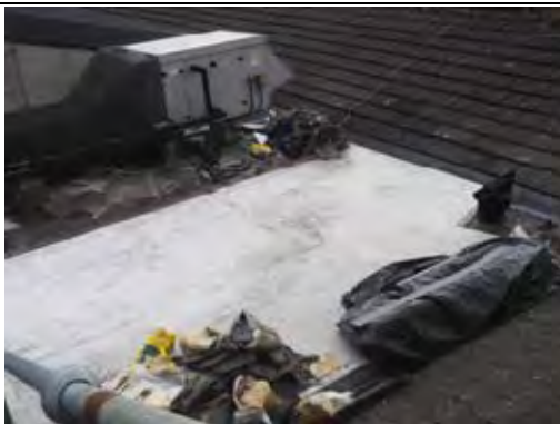
General view of roof. Insulation board debris CDCOTR/2 NADIS
