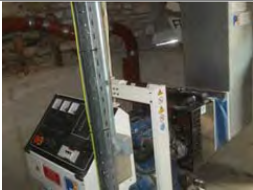
Modern non ACM boiler and exhaust
