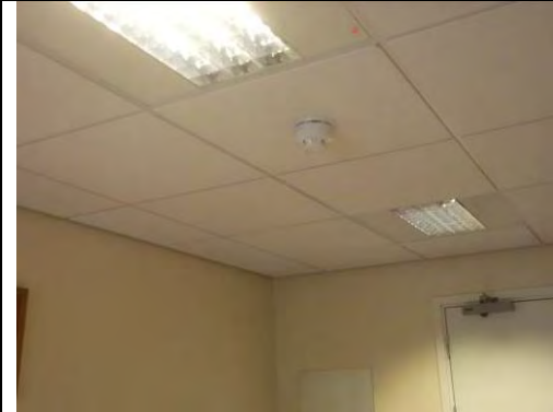
Modern non ACM suspended ceiling tiles and painted plastered and painted plasterboard walls
