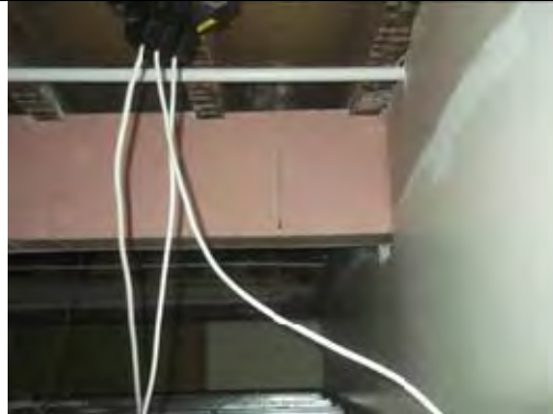
General view above suspended ceiling with modern non ACM fire resistant plasterboard to beam
