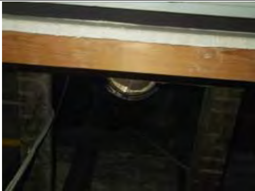
MMMMF to flue
