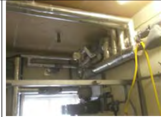
MMMFM and foil wrap to pipes. Non ACM
