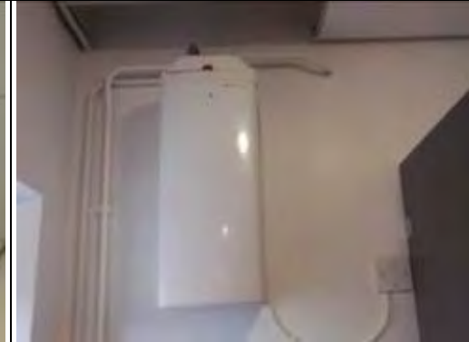
Modern non ACM water heater
