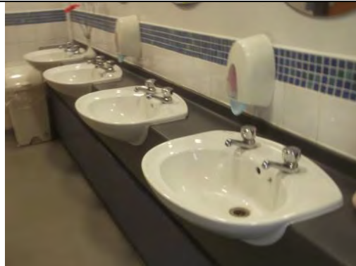
Modern non ACM sink units
