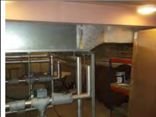
General view of Boiler Room
