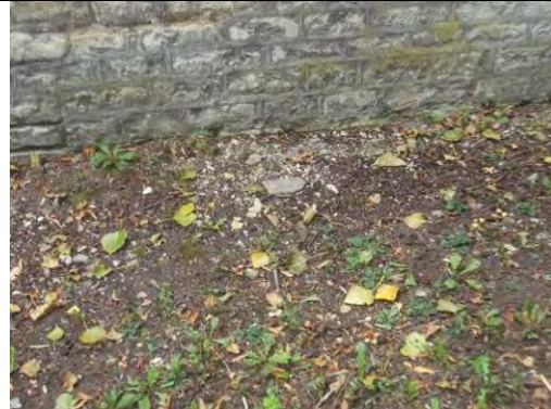
Asbestos cement debris within Garden. Removed
