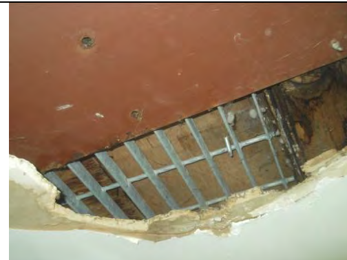
Landing. Painted plastered ceiling with original roof walkway over boarded above
