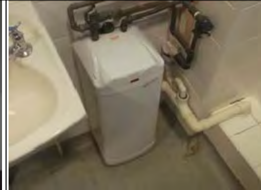
Modern non ACM water heater
