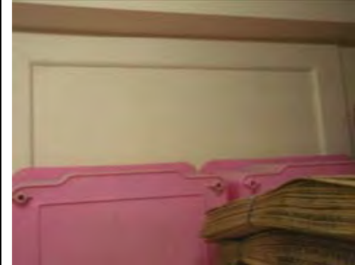
Non ACM panel to wall
