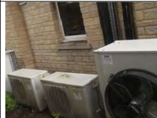
Modern non ACM air conditioning units
