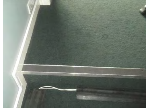
Carpet on concrete. Modern non ACM stair nosings
