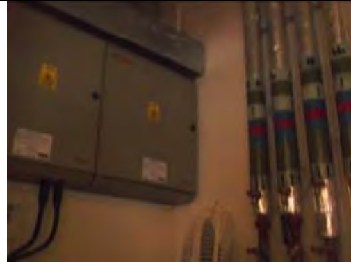
Modern non ACM electrics
