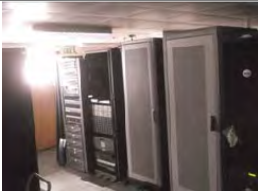
General view of 1.67 Server Room
