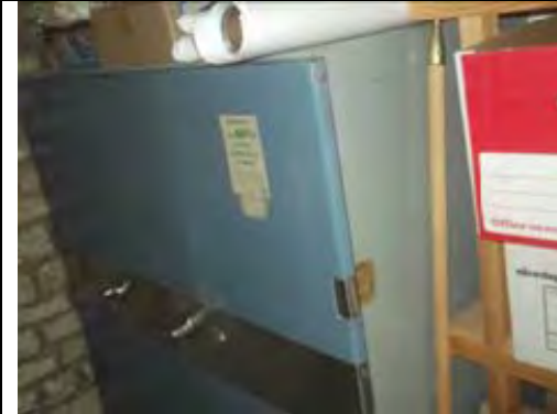
Presumed asbestos insulation board laminate to safe Crocidolite
