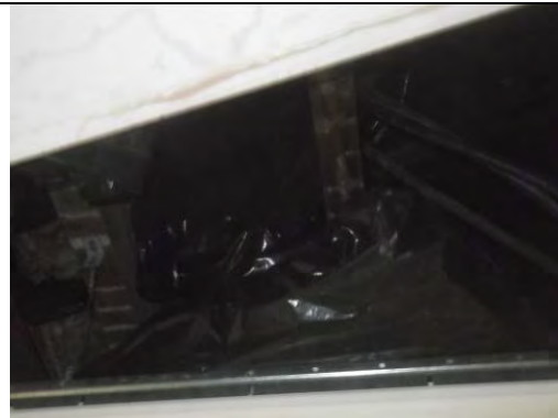
General view above suspended ceiling tile with MMMF insulation within black bags
