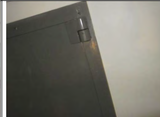
General view of 0.26 Strong Room with Strongly Presumed Asbestos steel laminate fire door Crocidolite
