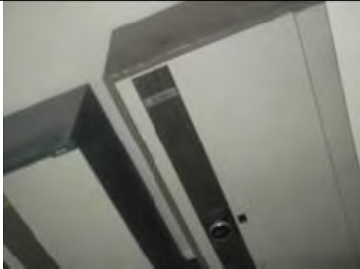
Presumed asbestos insulation board laminate to safes in corridor Opposite 0.25 / 26 Crocidolite
