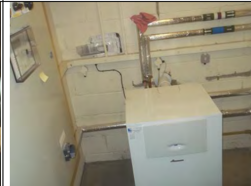
General view of 1.69 Boiler Room with modern non ACM boiler
