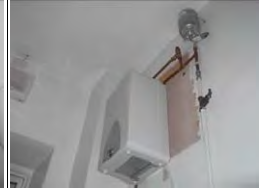
Modern non ACM water heater
