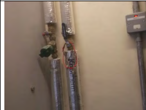
MMMMF insulation with foil wrap to pipes. Non ACM
