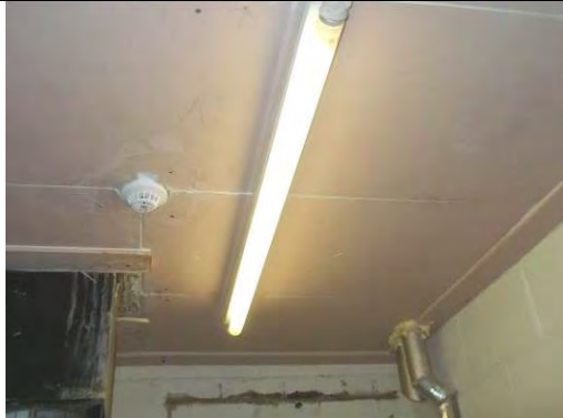
Fire resistant plasterboard ceiling
