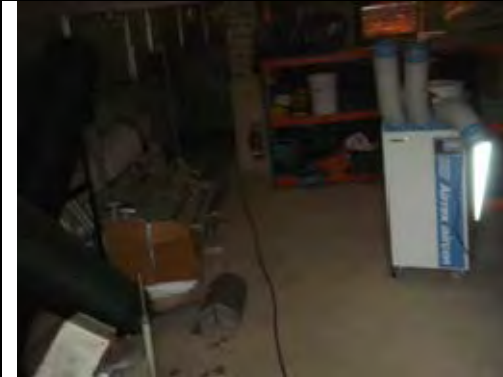
General view of Boiler Room
