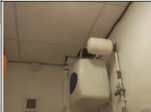
General view of Gents WC with modern non ACM electric water heater
