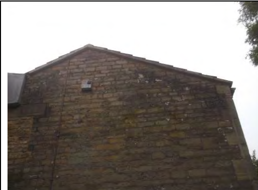
Cement under cladding to roof CDCOTR/1 Chrysotile
