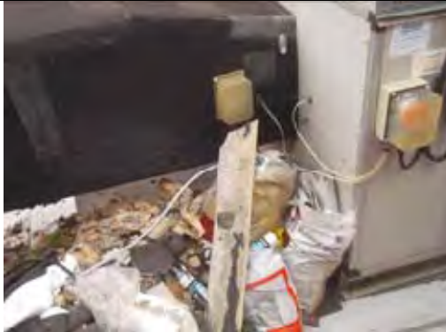
Asbestos cement debris. Now removed
