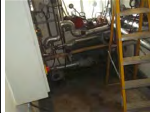
General view of Boiler Room
