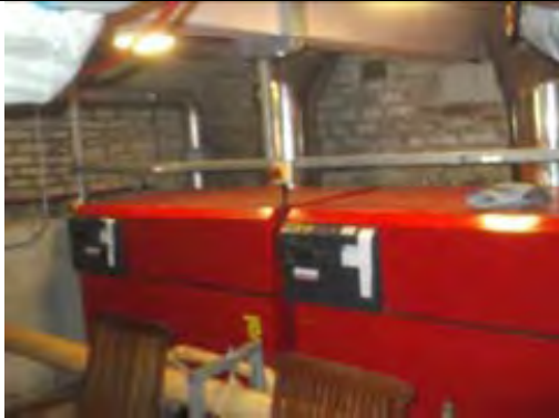
General view of Boiler Room with modern non ACM Boilers
