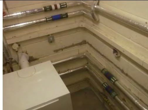
Foam and foil wrap to pipes. Non ACM
