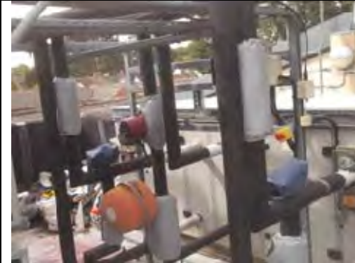
Modern non ACM pipe wrap to air plant
