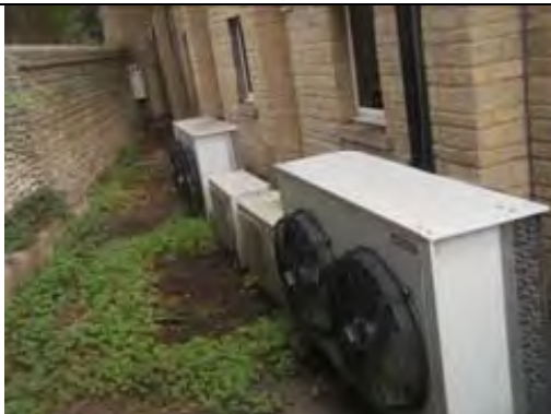
Modern non ACM air conditioning
