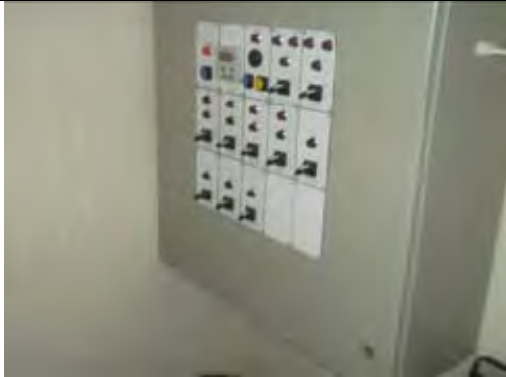
Modern non ACM electrics
