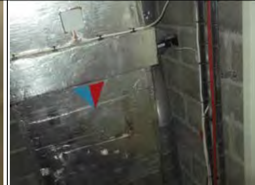
General view of Plant Room with modern non ACM insulation to plant
