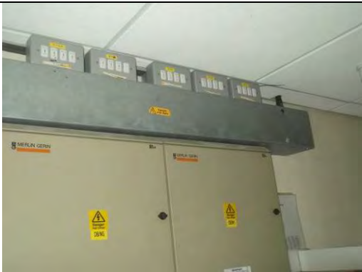
Modern non ACM electrics
