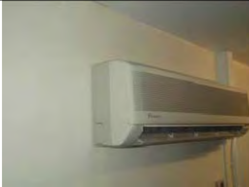
Modern non ACM air conditioning
