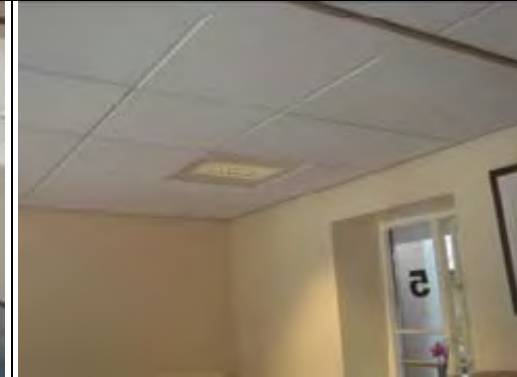
Modern non ACM suspended ceiling tiles and painted plastered and plasterboard walls
