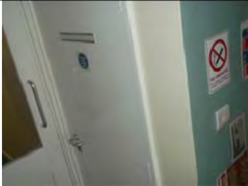
No Access to understairs cupboard
