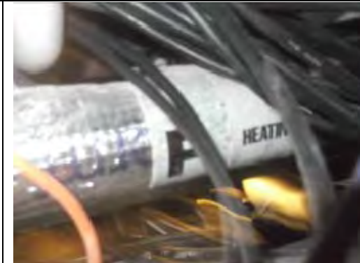
Modern non ACM heating pipes
