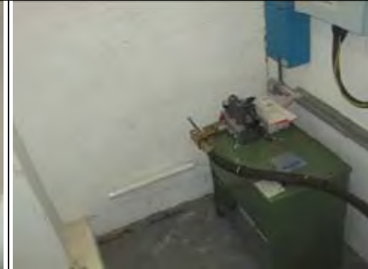
General view of 0.5. Lift Motor Room
