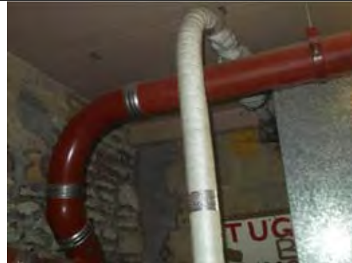
Modern non ACM wrap to exhaust pipes
