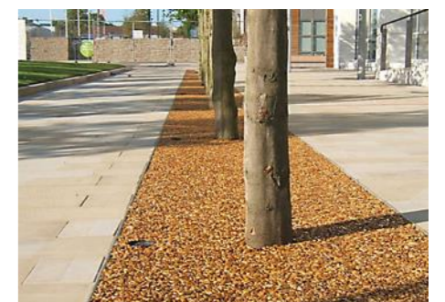
Figure 3.50: Porous resin bound gravel tree pit surfacing. Image shows 'Addastone TP' from Addagrip
