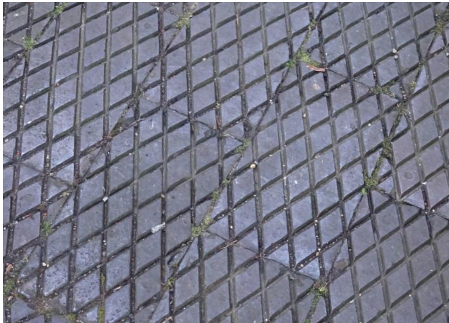
Figure 3.7: Diamond chequered blue brick pavers is widely used in front gardens on Ashcroft Road
