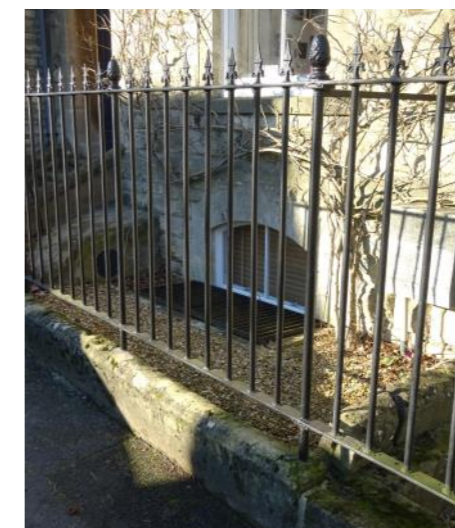
Figure 3.56: Metal Railings on top of a low stone wall on The Avenue
