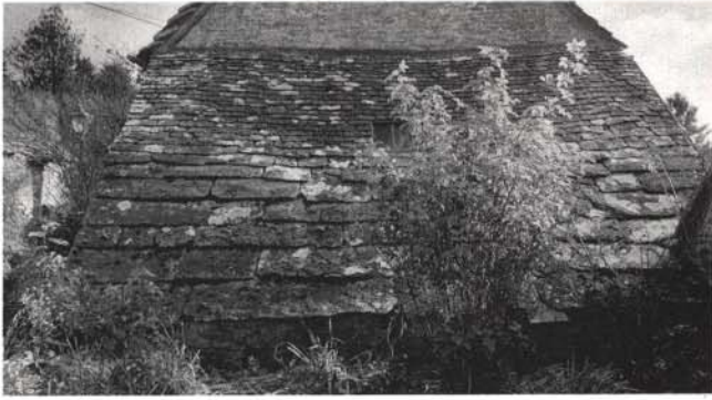
Almost all of Chedworth's old buildings are roofed in natural stone slates. This roof, on an outbuilding near Amphlett House, has some unusually large specimens in the lower five courses.
