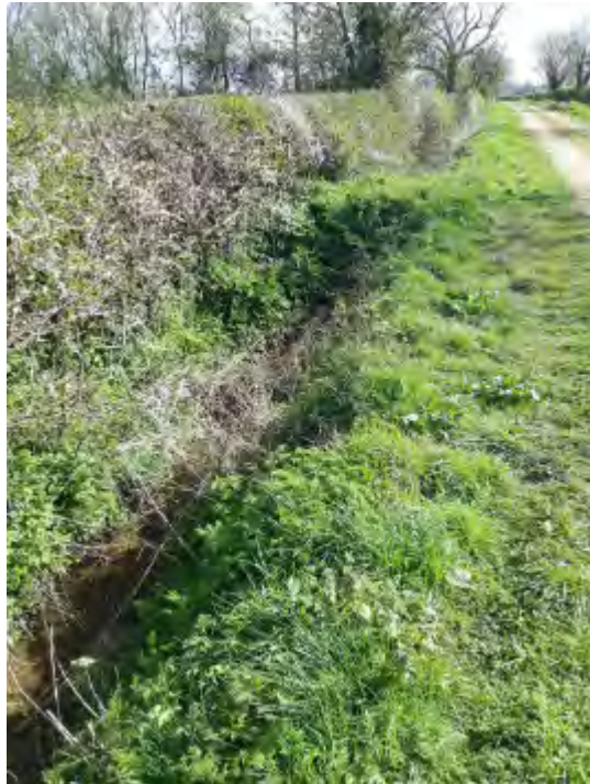
Photograph 2 - Drain B1 Looking south showing obstruction (2020).
