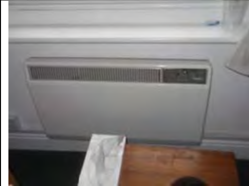
Modern non ACM electric heater
