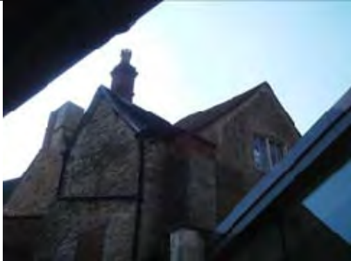
Presumed asbestos cement undercloaking to verge edge of roof
