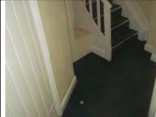
General view of Stairs leading to Room 3 with modern non ACM stair nosing
