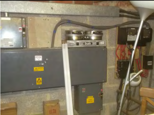
Modern non ACM electrics
