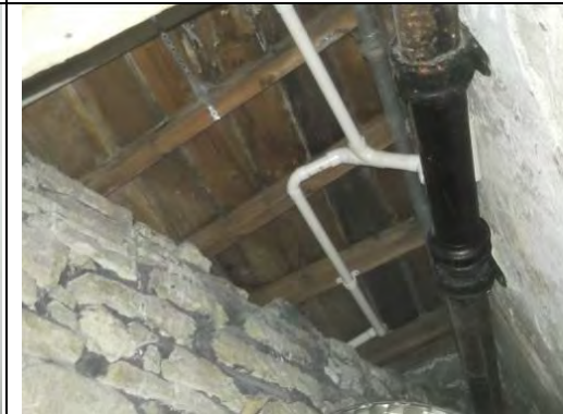
Presumed asbestos rope seals to spigot joints of cast iron pipes
