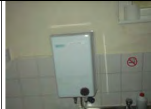
Modern non ACM water heater
