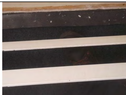
Insulation board AHC/1 Amosite/ Chrysotile
