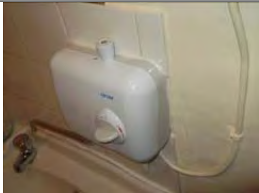
Modern non ACM water heater
