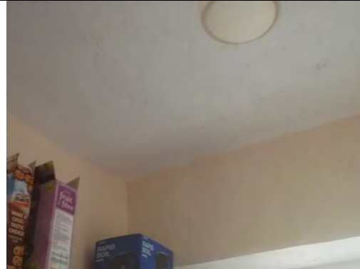
Textured coating to ceiling AHC/4 NADIS
