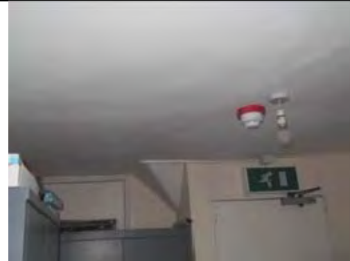
Painted plastered walls and ceiling and non ACM insulation board to door AHC/6 NADIS
