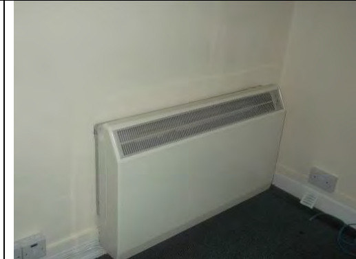
Presumed asbestos insulation board, ropes and seals to heater Crocidolite
