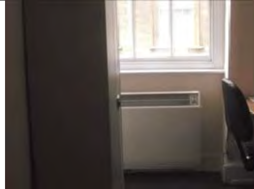
Presumed asbestos insulation board, ropes and seals to heater and board behind Crocidolite
