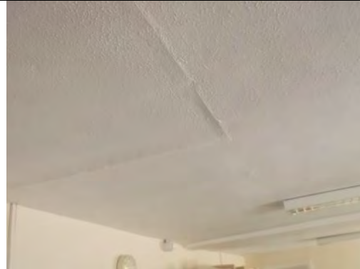
Textured coating to ceiling AHC/3 Chrysotile
