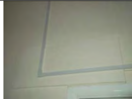
Insulation board above door AHC/8 NADIS
