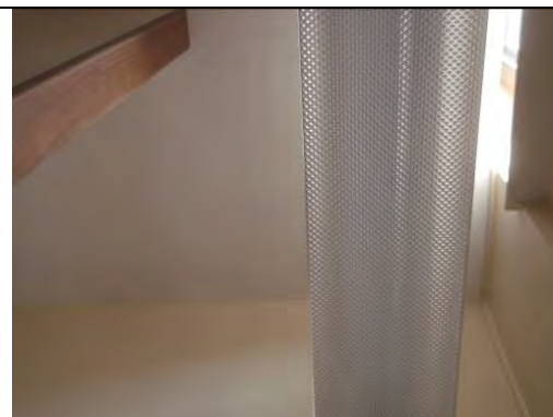
Insulation board to ceiling VS to AHC/1 Amosite/ Chrysotile
