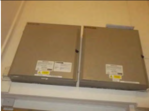
Presumed asbestos flash guards, ropes and seals to electricians Chrysotile
