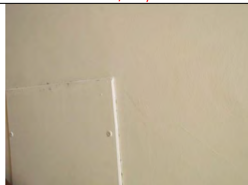
No ACM panel to wall
