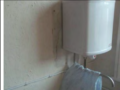
Modern non ACM water heater
