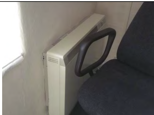
Presumed asbestos insulation board, ropes and seals to night storage heater Chrysotile
