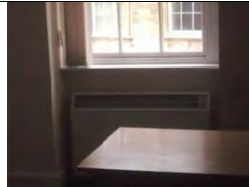
Presumed asbestos insulation board, ropes and seals to heater and board behind Crocidolite
