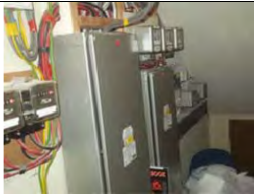
Presumed asbestos flash guards, ropes and seals to electrics
