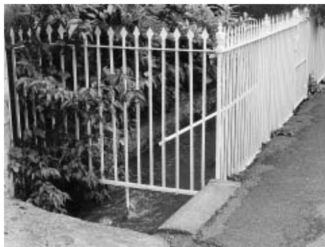
These boundary railings in Lower Street, with their fine detailing, enclose a short length of stream in an unusual manner. These features contribute to the character of Blockley and need careful conservation.
