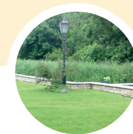
5. At Gas Lane a sheet-piled wall, earth bund and a low-level flood wall were built. This reduces flood risk to Gas Lane and Back Lane.
