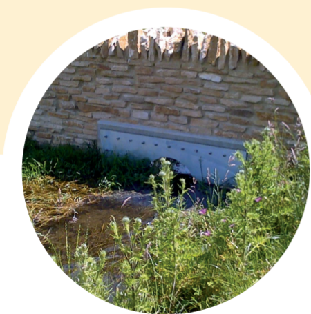
2. At Milton Street a flow control structure was built across Waterloo Brook. This protects Milton Street and cuts off the flow of water onto London street.
